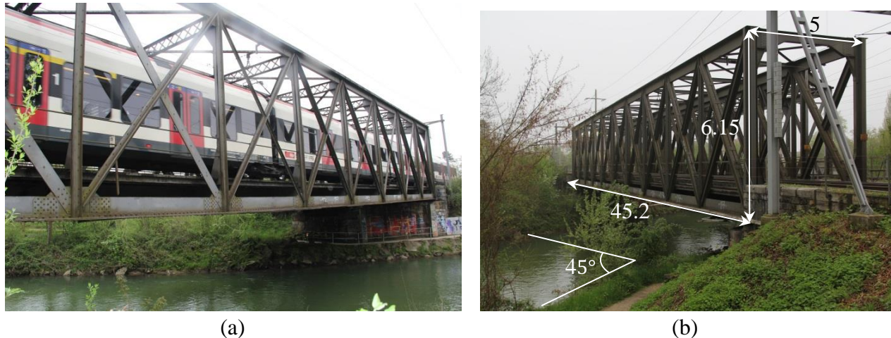
Fig. 3.7.5. Münchenstein railway bridge (a) subjected to an S3 train, (b) consists of 10 panels with the total length of 45.2 m, width of 5 m and height of 6.15 m, built on a 45-degree skew.
